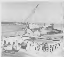
NOW YOU SEE IT — A multi-ton steel wrecking ball swings from the giant arm of F-6 crane to reduce to rubble the old Plant Dispensary located on the main road near the General Shops.
